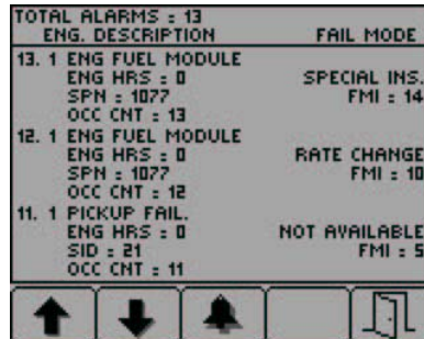
Figure 7.8.3: The alarm list screen, showing that alarm conditions have been acknowledged. Note that the exit key (key #5) has now been activated.
