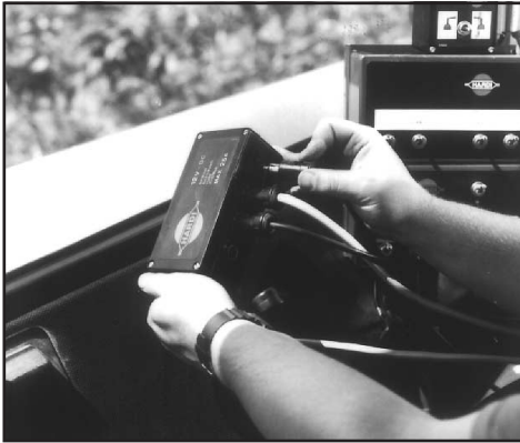
Fig. 16 (12-volt junction box for 12-volt hook-up for EC controls, foam marker, boom hydraulic controls, etc)
